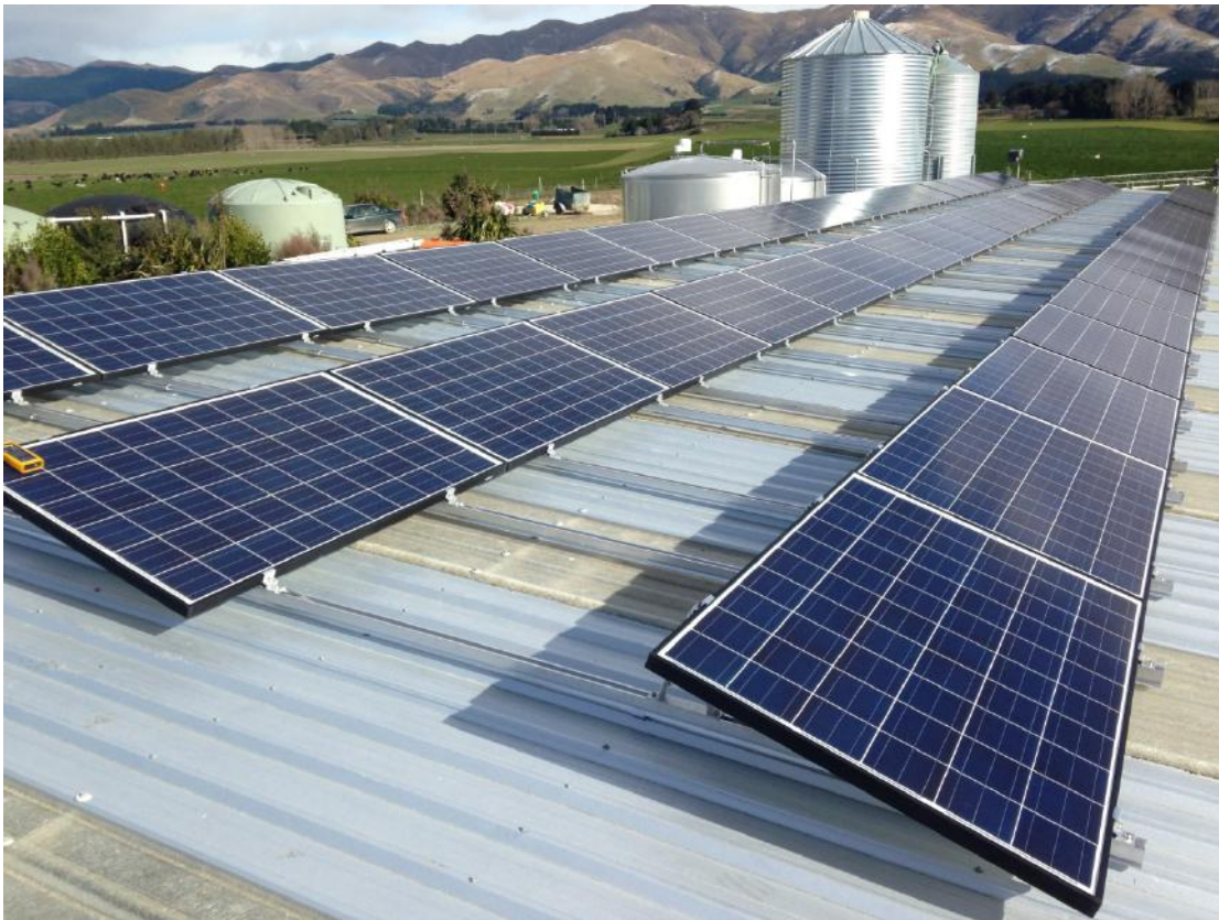
Figure 3.22 Solar array on a dairy shed near Waimate
