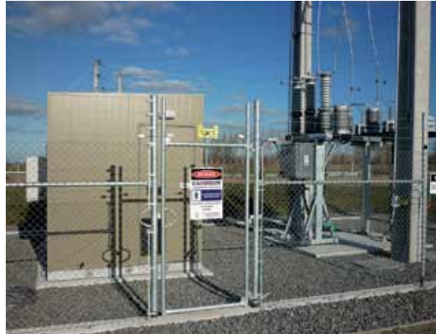
New Canal Road Substation
